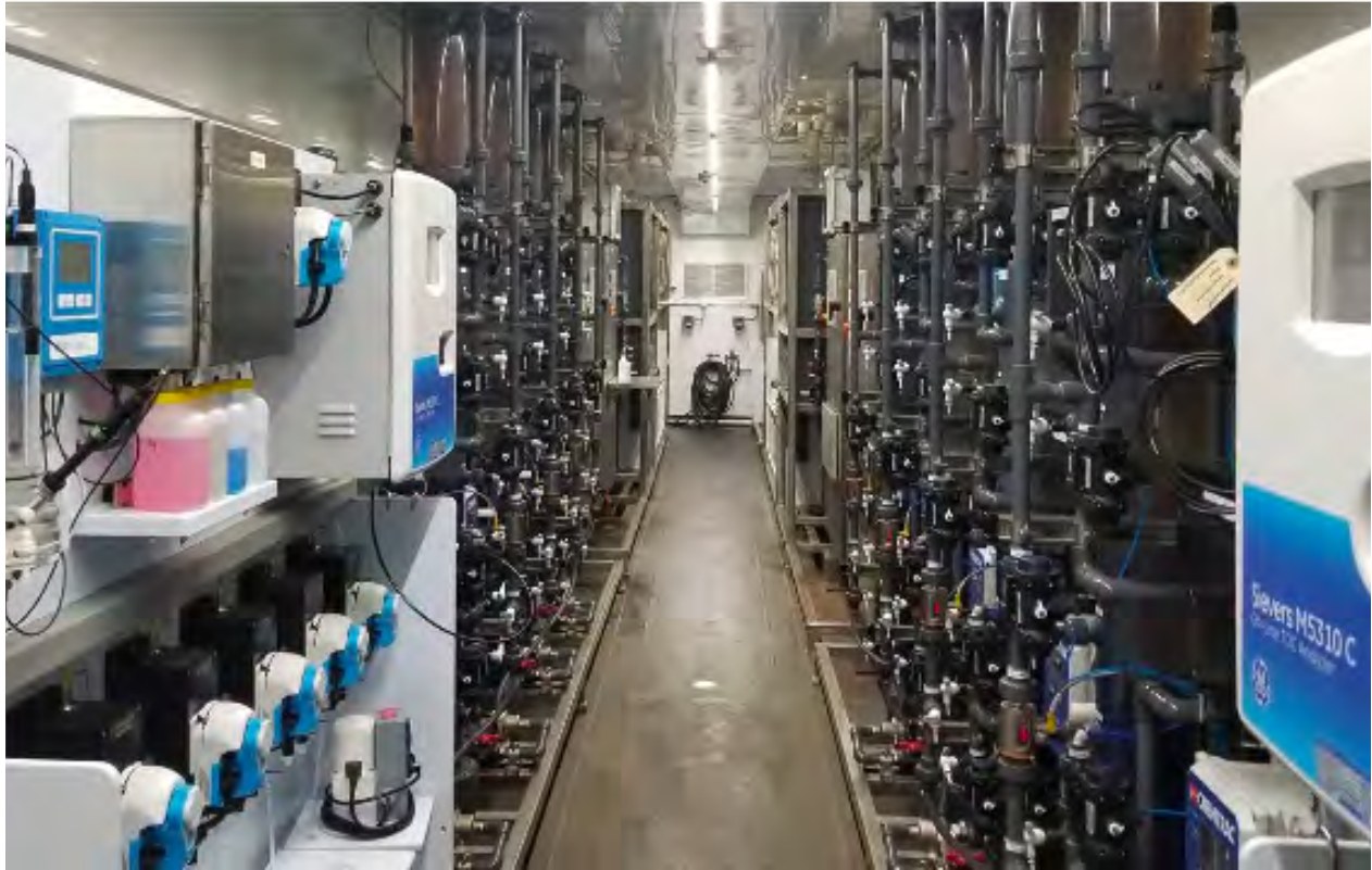
BWW'S MOBILE PILOT PLANT TESTS WATER PROCESS TREATMENT ALTERNATIVES.
