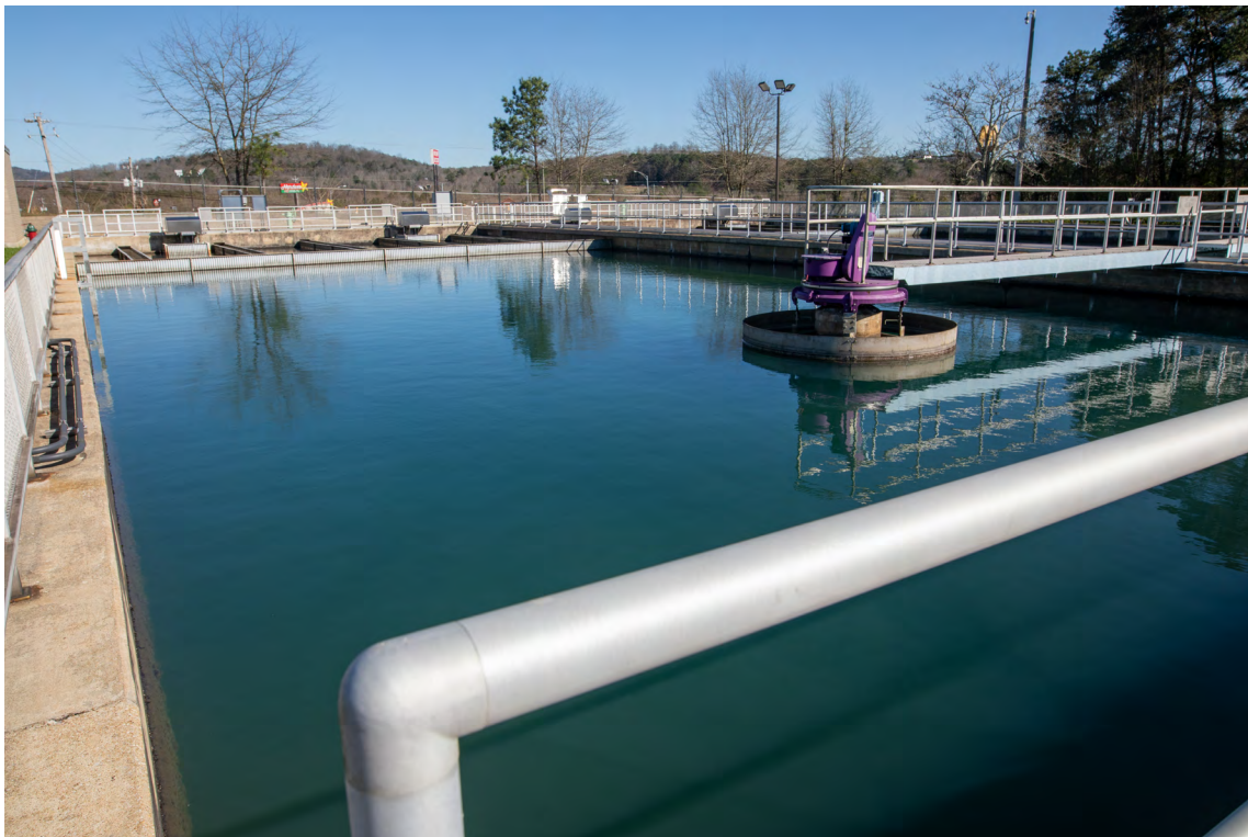
CARSON FILTER PLANT
